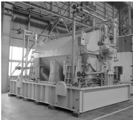
Fig. 7 Cracked Gas Compressor (荏原エリオット)
